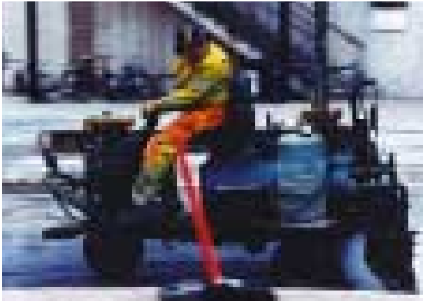
Active product development provides customer value. NCC has a long track record of developing and refining products for paving work.
